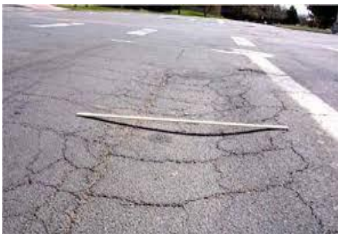
Figure 1. Degradations of Rutting in road
